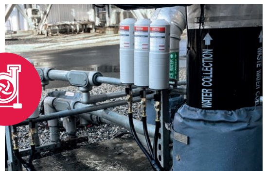
Industry: Power Generation Application: Pumps
